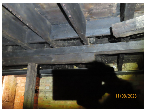
Failed timber supports
