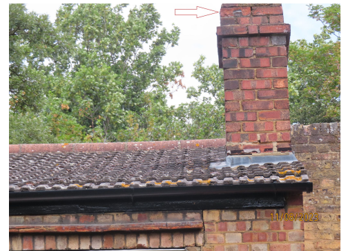
Evidence of spalled brickwork
