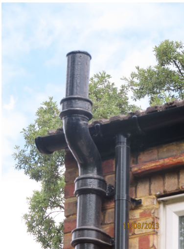
Soil and vent pipe
