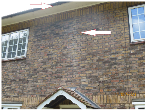
Staining to brickwork and potential leak to gutter joint.
