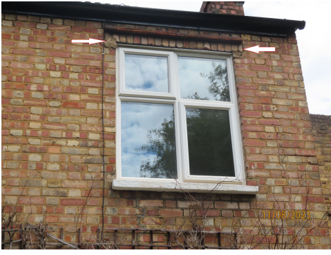
Movement to brickwork soldier course.
