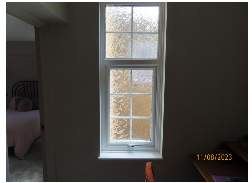
Low level window to landing
