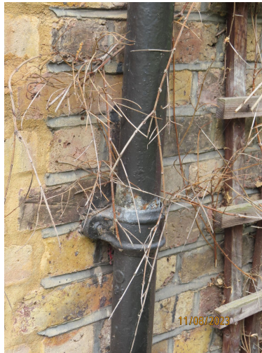
Corrosion and leaking around downpipe join.
