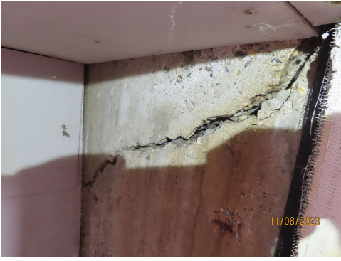
Crack in retaining wall near access hatch
