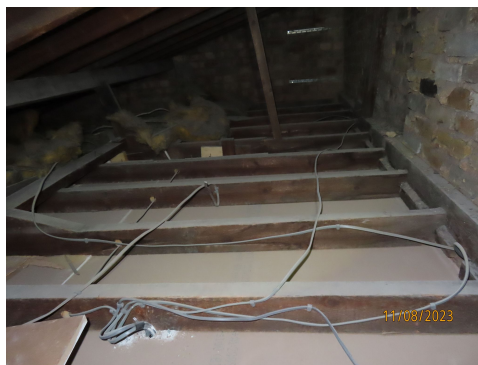
Lack of insulation to the roof space
