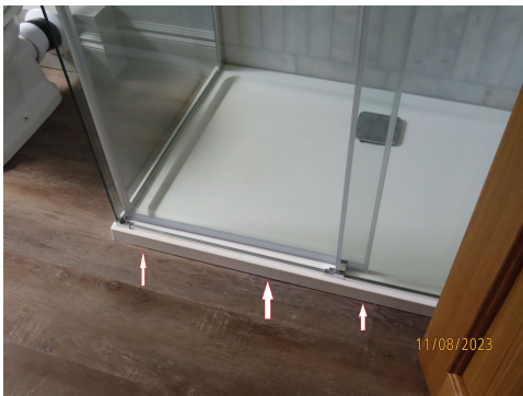
Missed mastic seal to shower tray.
