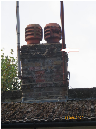
Vegetation to chimney stack
