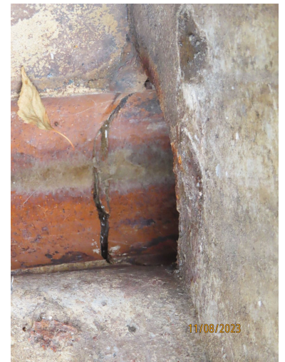
Cracked drain to rear
