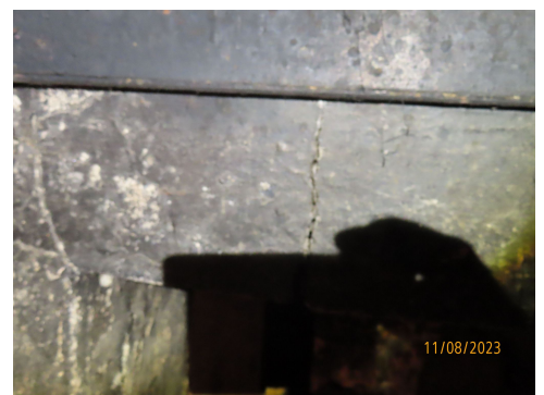
Cracked lintel support to fireplace.
