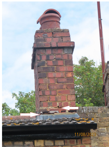
Worn pointing to mortar joints
