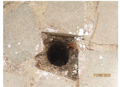
Hole in paving to rear patio
