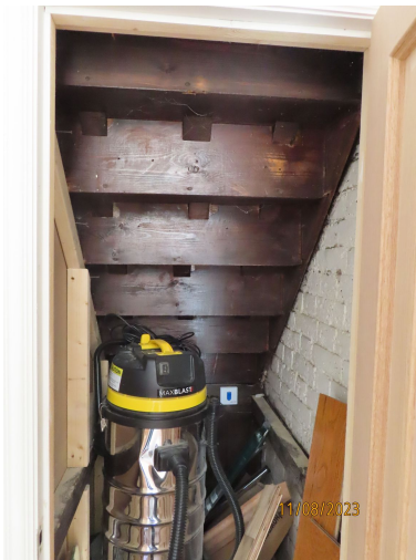
Lack of fire protection to staircase
