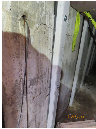
Timber supports showing signs of bowing.
