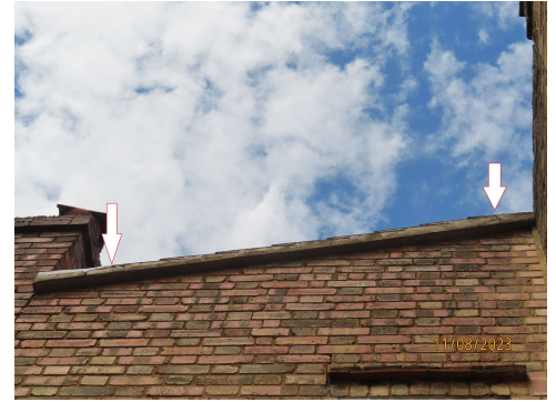
Light cracking to mortared verge
