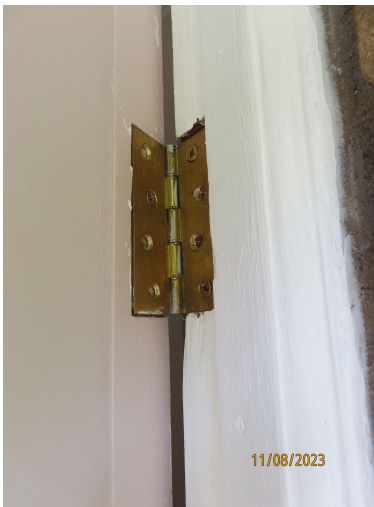
Missing screws to front door.
