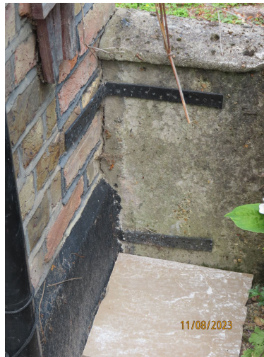
Restraint straps to front boundary wall.
