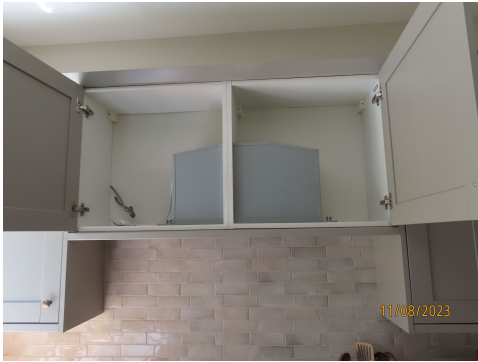
Kitchen extractor not connected.
