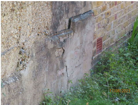
Bulging and cracking to front boundary wall.
