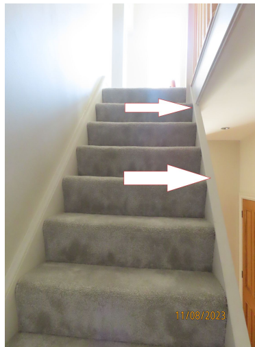
Lack of banister or balustrades to staircase.
