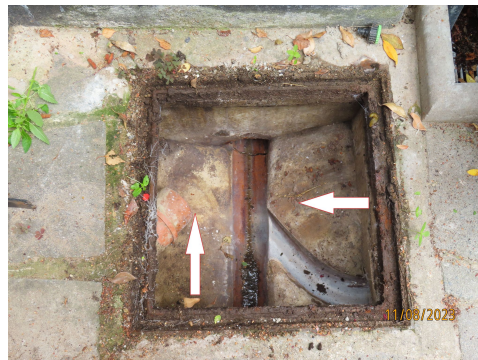
Rear inspection chamber. Arrows indicate direction of flow.
